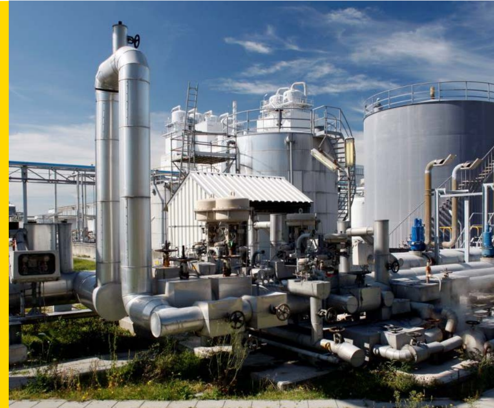
Botlek Steam Pipe
